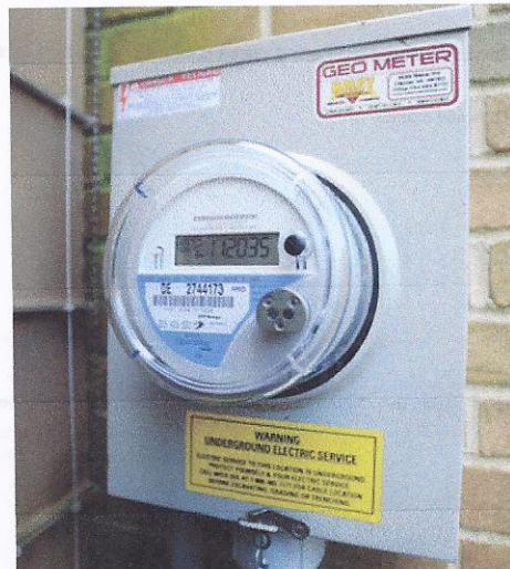
A DTE smart meter installed at a local residence.
